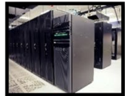
Corporate Research and Development Server Facility (CRDSF)
