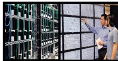
High Performance Computing Facility
