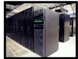
Corporate Research and Development Server Facility (CRDSF)
